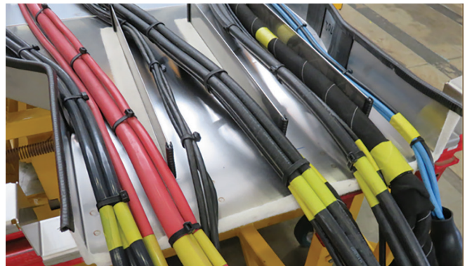
Figure 28: Typical electrical cables.
