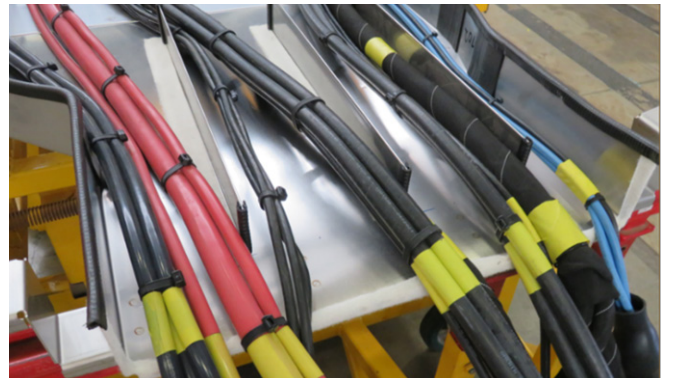
Figure 28: Typical electrical cables.
